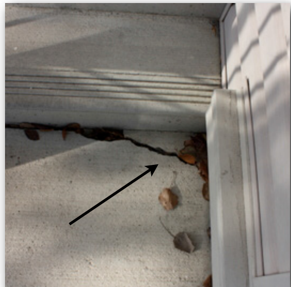
3.12 Settlement at the stairs of Unit 67.
