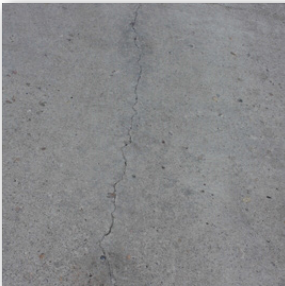
3.7 Some cracking in concrete driveway aprons.
