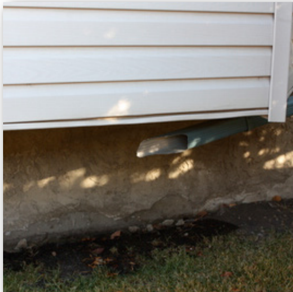
3.1 Downspouts located too close to the foundation of the building.
