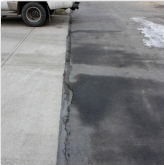
3.9 The joint between driveways and pavement is in need of new sealant.
