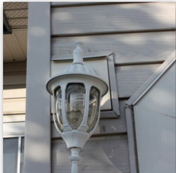
3.6 Standard exterior light fixtures.
