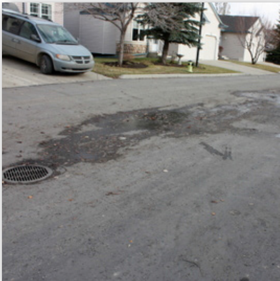
3.11 Settled area in the asphalt pavement resulting in poor drainage.
