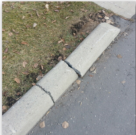
3.8 Break offs to the cast in place concrete curbs.
