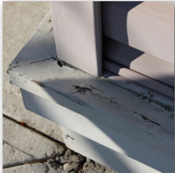
3.2 Extensive peeling of paint on wood trim.
